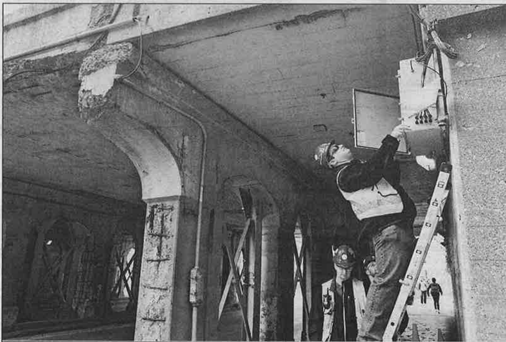
Research Engineer Mat Kotowsky finishes work on a wireless transmitter, which is part of a system of stress sensors on the CTA viaduct over Sheridan Road near Devon Avenue. CHRIS WALKER/TRIBUNE PHOTO
