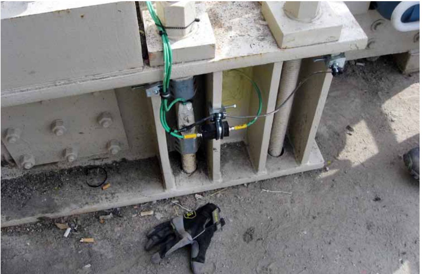
The ITI-developed clamped strain sensor for threaded rods deployed on the Kennedy Bridge bearing retrofit.
