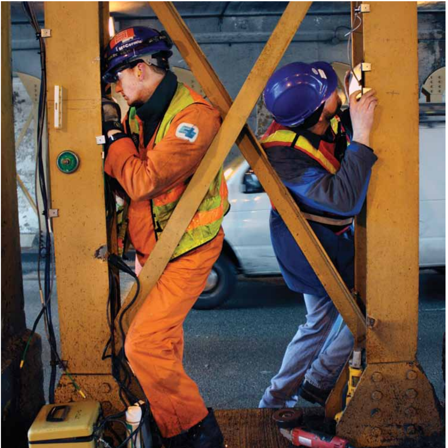
ITI Research Engineer David Kosnik (left) and Prof. David Corr (right) install strain gages on steel columns at the Devon-Sheridan overpass.
