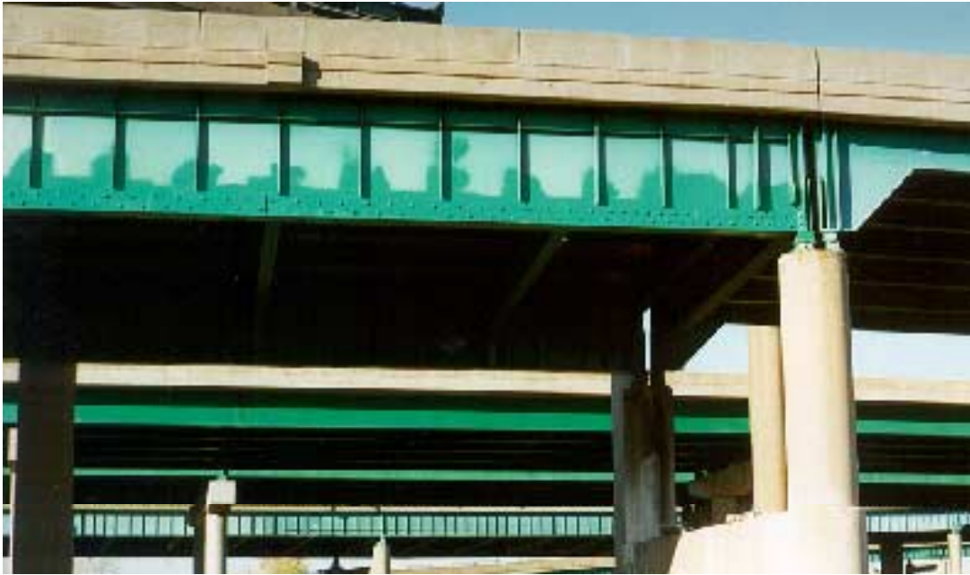
Figure 12. Retrofitted I-55/I-64/US-40 Poplar Street Bridge Complex over the Mississippi River, St. Clare County, Illinois
