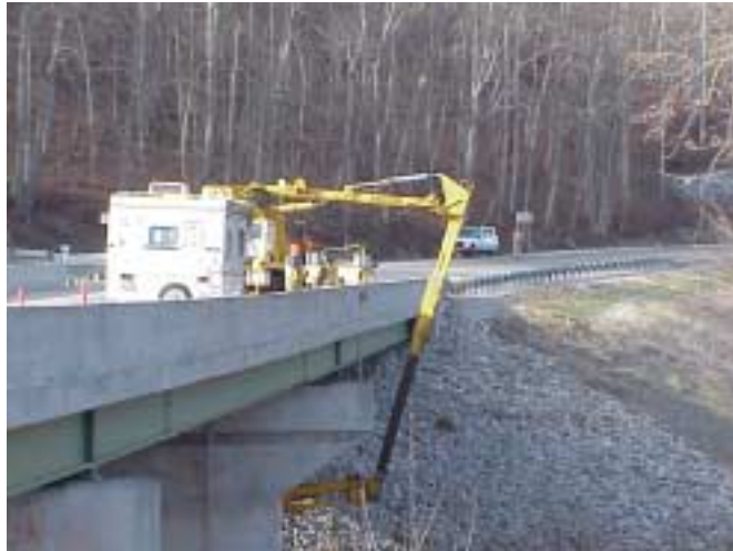
Figure 16. Remote Monitoring System Installation, SR62 Bridge over Little Blue River, Crawford County, Indiana
