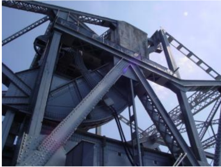
Rack and Pinion Support Structure, Michigan Street Bridge, Sturgeon Bay, WI
